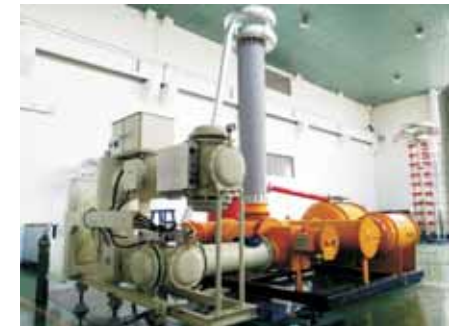
1200kVA/600kV test system with universal adjustable platform
